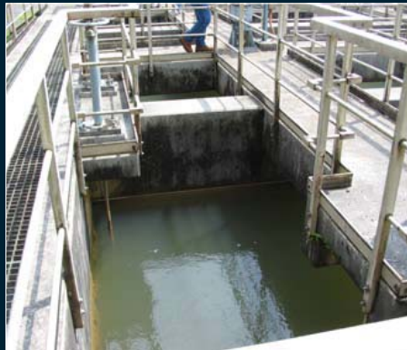
Koror-Airai Treatment Plant, Koror, Palau
